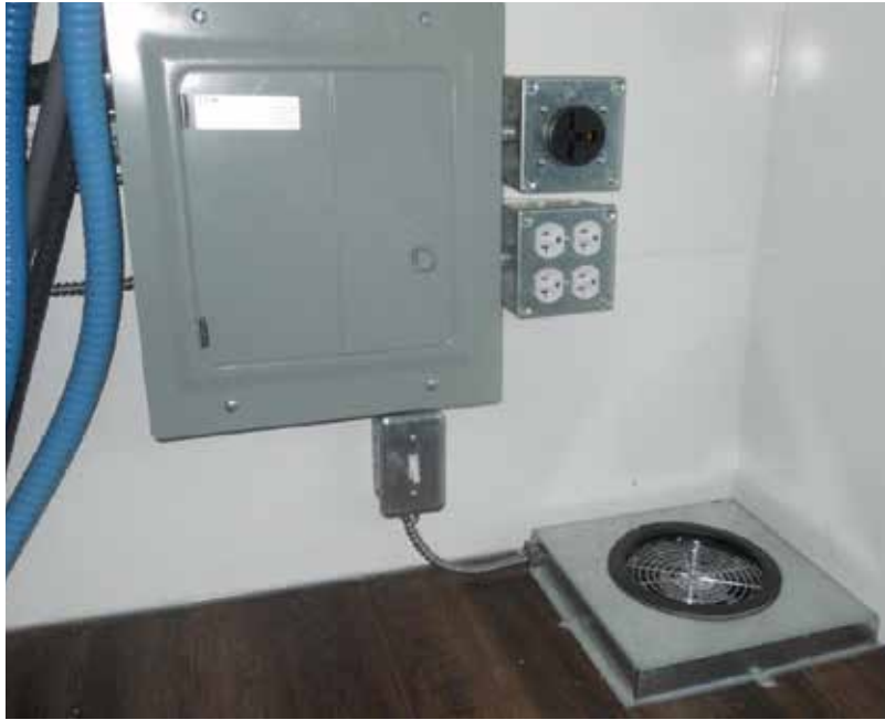
Electrical Breaker box with convenient 110-220 volt outlets.
