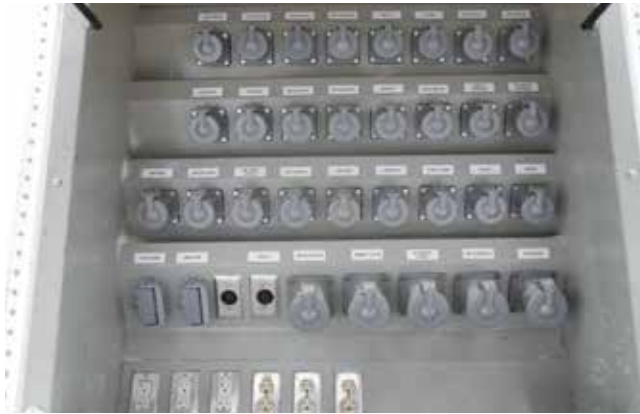
Electrical plug box. Electrical box door is closed when in operation, Cords go out bottom.
