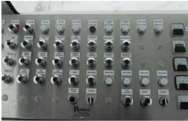
Pre-wired Stainless steel console to accommodate 55 stations.
