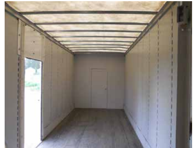
Insulated partition wall with door between generator and MCC room.
