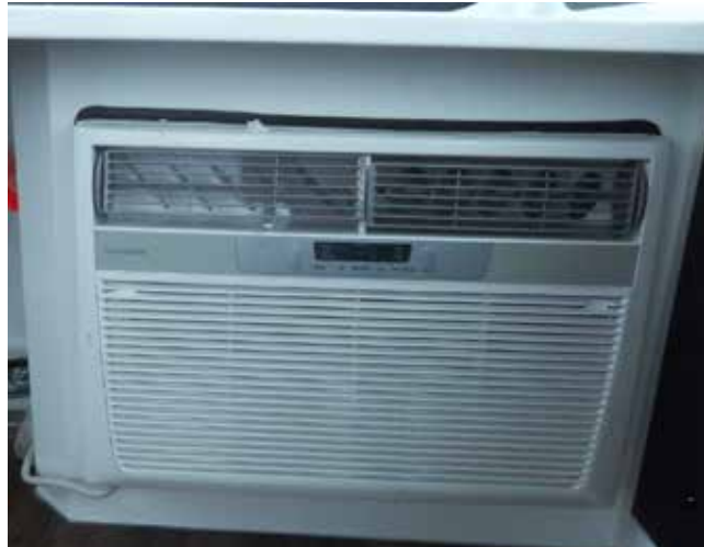
Oversized 25,000 BTU A/C & Heater unit Pulls clean air from inside trailer.
