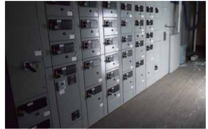
Switch gear installed in trailer.
